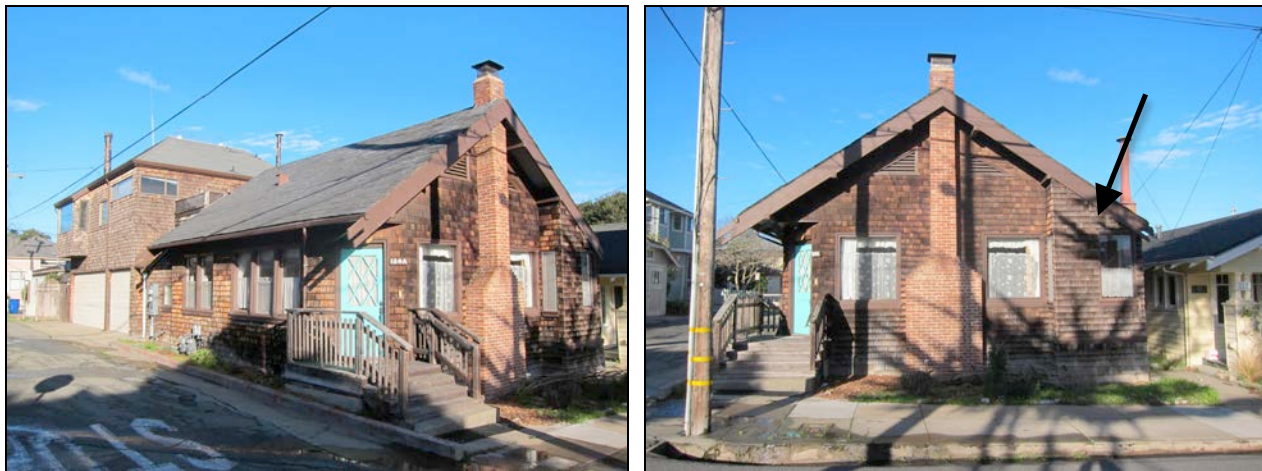
Figures 2 and 3. Left image shows the east and south elevations with the large, two-story circa-1971 addition toward the far left. Right image shows the east elevation on 17 th street. The original porch was on the northeast corner (arrow).
